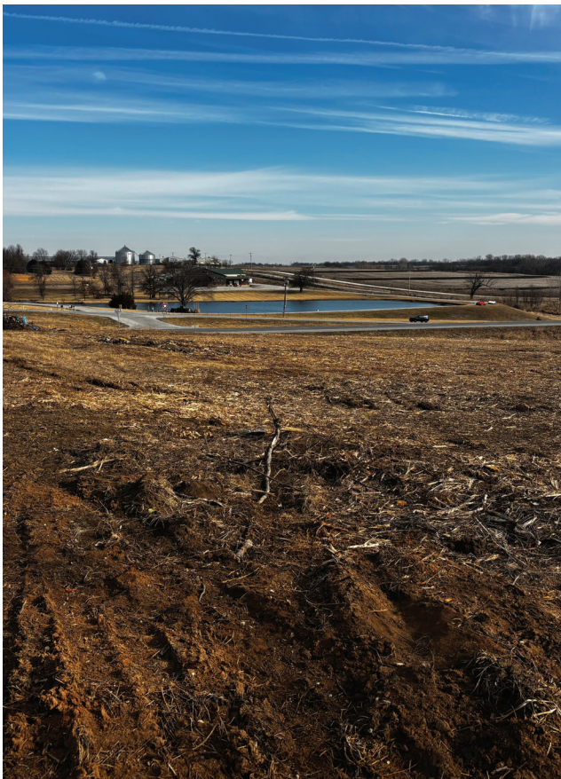
(Top and above) Site work has begun for the new Lone Jack Substation, which will support current and future growth in this developing area of WCE co-op country.
